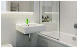
Control flow taps
